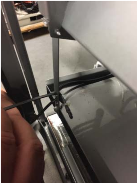
Figure 10. Relocate T-1 Sensor
