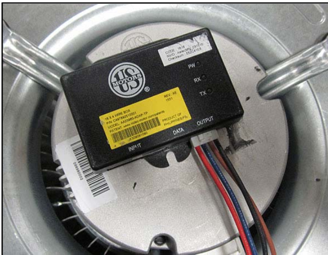
Figure 12. Black Box Repositioned on Motor Module
