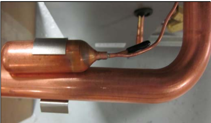
Figure 26. External Suction Line
