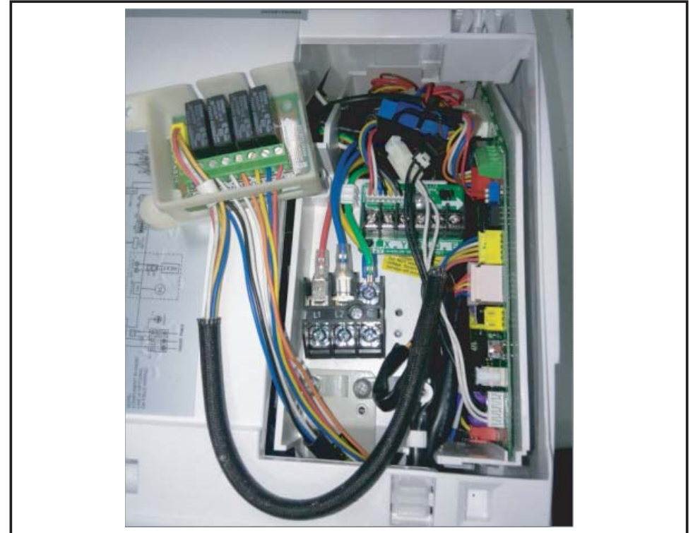
Figure 14. VWMA007-018 Install Inside of Control Box
